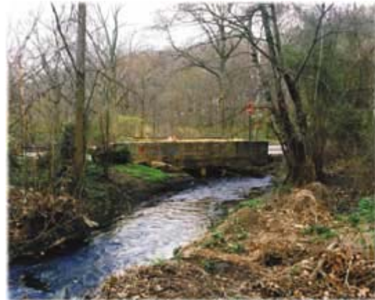
Before: structurally deteriorating undersized culvert at Aultman Avenue
