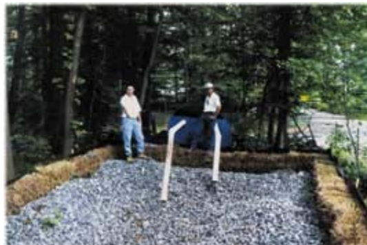
The deputy director of the Bluebelt project (left) inspects proper functioning of the portable sediment tank with sediment trap.
